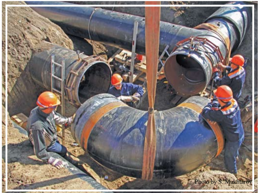
Mainline Pump Piping installation, Kropotkin PS
