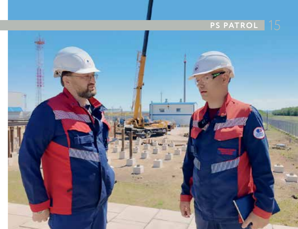
P. A. KRETOV AND D. R. ENALIEV AGAINST THE BACKGROUND OF THE CONSTRUCTION SITE OF VFD BLOCK BOXES AT PS 5
