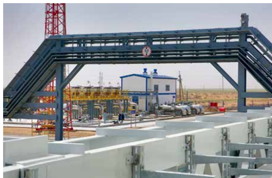
PRESSURE MITIGATING SYSTEM AT THE CPC FACILITY
