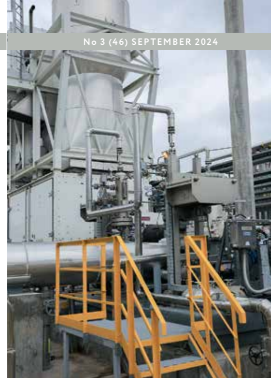
SAFETY HANDRAILS AT THE KROPOTKINSKAYA PS
